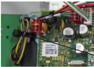
CONNECTION OF THE TOUCHSCREEN ON J3 BOARD
