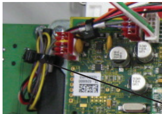
CONNECTION OF THE TOUCHSCREEN ON J3 BOARD
